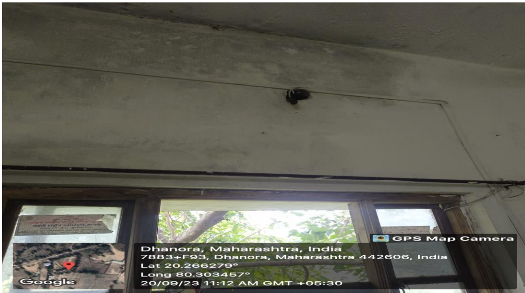
CCTV Cameras in the campus
